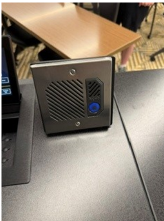
Algo 8201 intercom integrated into the lectern top
