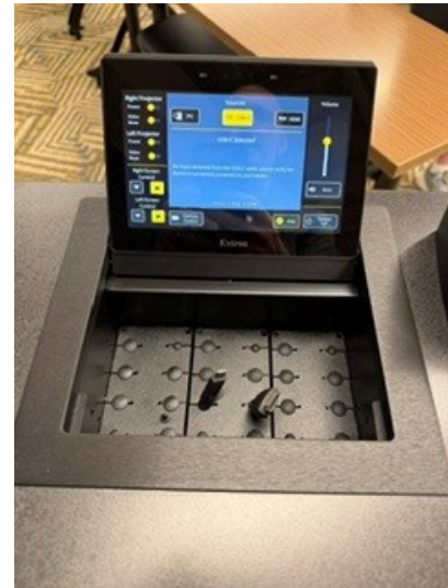
Extron 725 cubby with integrated controls
